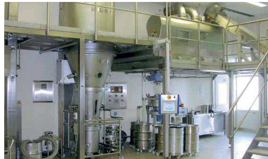
Pharmaceutical drying and coating system
